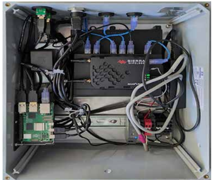
Prototype wall-mounted data collection server
